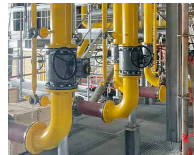
Pipe installation in the new energy center – hot water instead of steam in the „Weißenburger Straße“.
